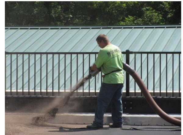
MCS Inc. worker installing growing media made from compost on green roof. www.mcsnjinc.com
