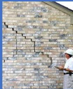
A house built in expansive soils
